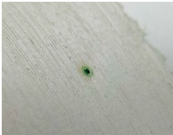
An extreme close-up of the burn mark at the first layer of insulation. Notice where the ionized copper left a green-colored mark.
